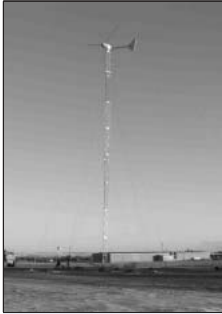
Liberty County's newly built 10 kW, the third Montana turbine installed as part of Our Wind Co-op. Photo credit: Don Marble
